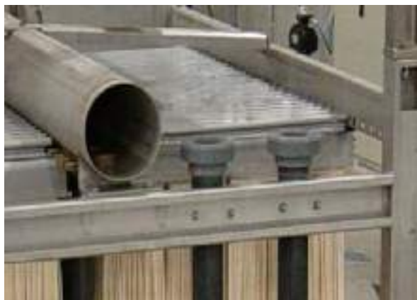
figure 5.6 - aeration unions installed
