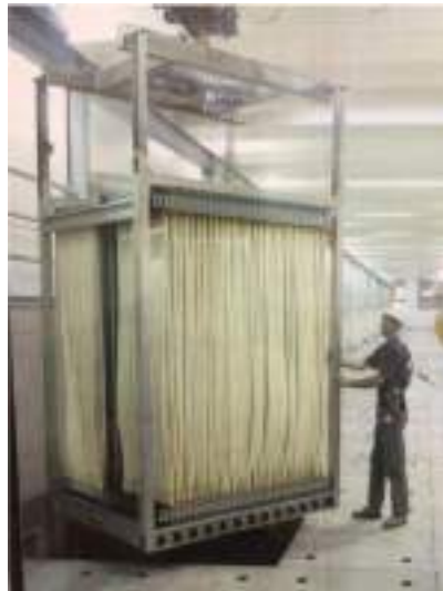
figure 5.16 - membrane tank with FRP cover
