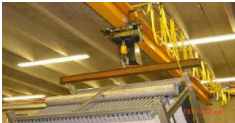
figure 5.10 - hoist with spreader bar
